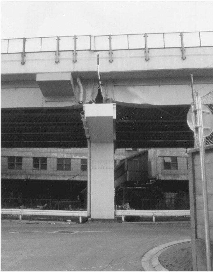
FIGURE 2.13 Girder damage at Bent 351 of the Hanshin Expressway apparently due to transverse movement during the 1995 Hyogo-Ken Nanbu earthquake.
