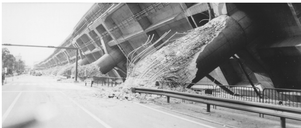
FIGURE 2.4 Higashi-Nada Viaduct collapse in the 1995 Hyogo-Ken Nanbu earthquake. (Source: EERI, The Hyogo-Ren Nambu Earthquake, January 17, 1995, Preliminary Reconnaissance Report, Feb. 1995.)
