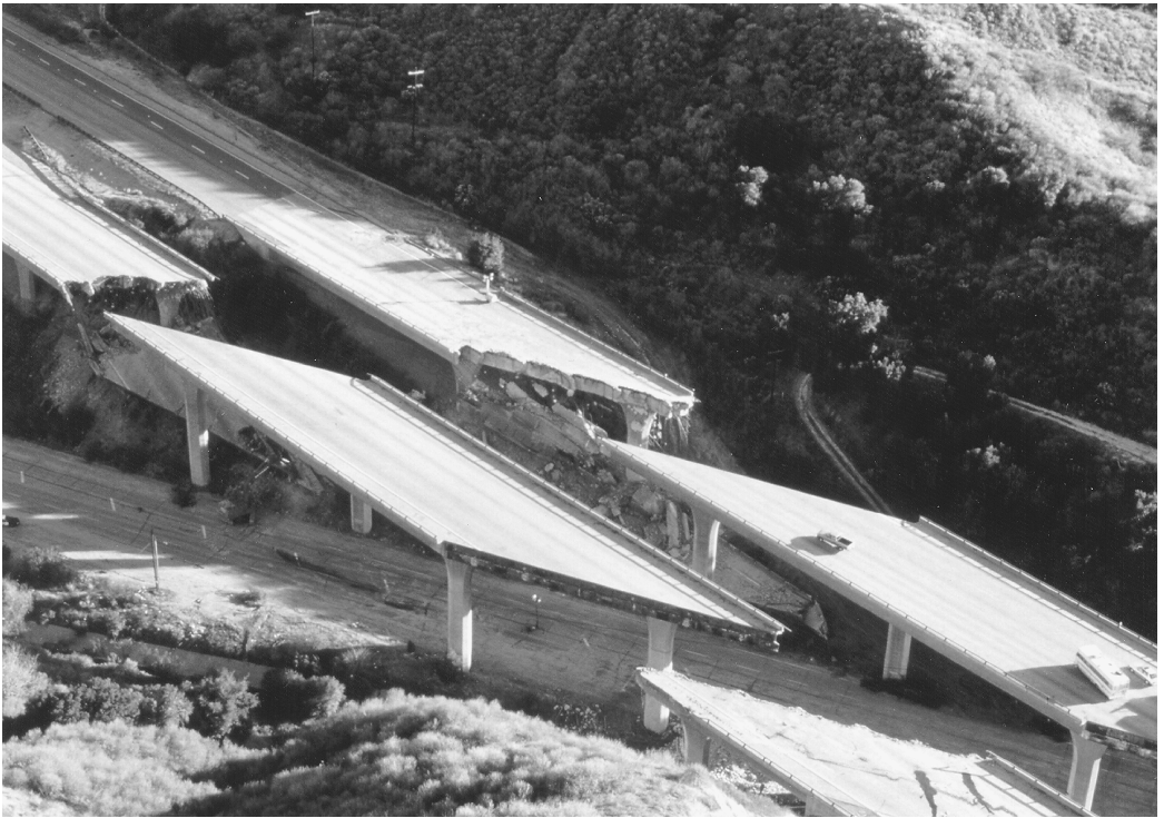
FIGURE 2.10 Gavin Canyon Undercrossing collapse in the 1994 Northridge earthquake.
