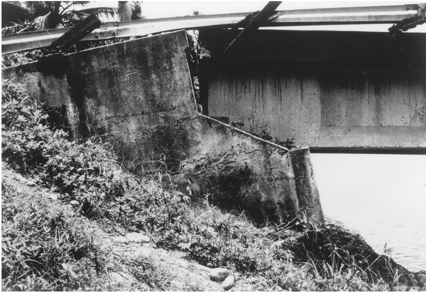
FIGURE 2.32 Rotation of abutment due to liquefaction and lateral spreading during the 1991 Costa Rica earthquake. (Source: EERI, Earthquake Spectra , Special Suppl. to Vol. 7, 1991.)
