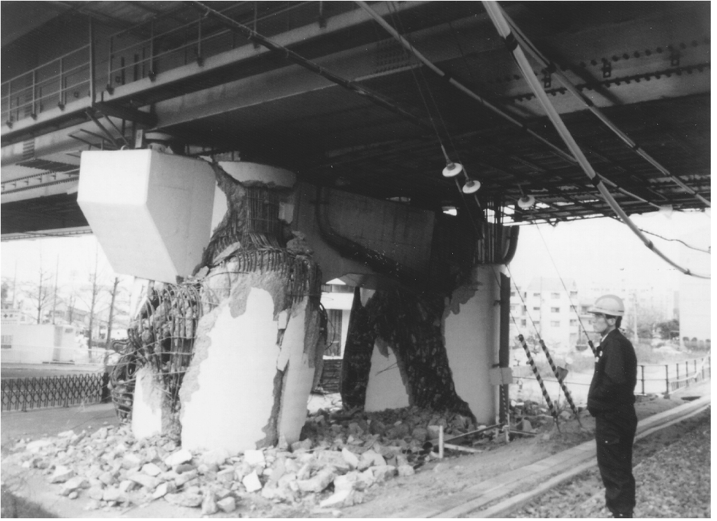
FIGURE 2.23 Failure of a two-column bent in the 1995 Hyogo-Ken Nanbu earthquake.
