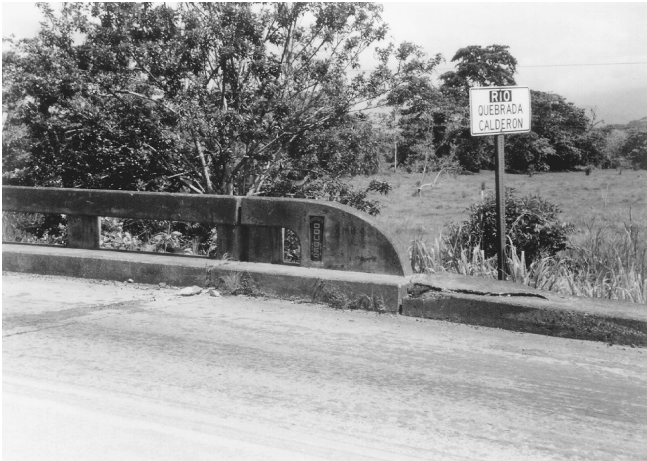
FIGURE 2.34 Settlement slab spanning across slumped abutment fill material at the Rio Quebrada Calderon bridge in the 1991 Costa Rica earthquake. (Source: EERI, Earthquake Spectra , Special Suppl. to Vol. 7, 1991.)
