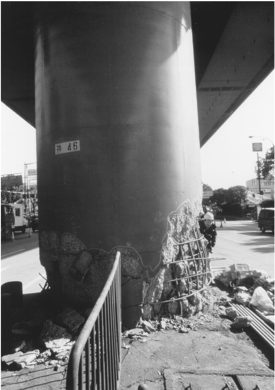
FIGURE 2.18 Hanshin Expressway, Pier 46, damage in the 1995 Hyogo-Ken Nanbu earthquake.
