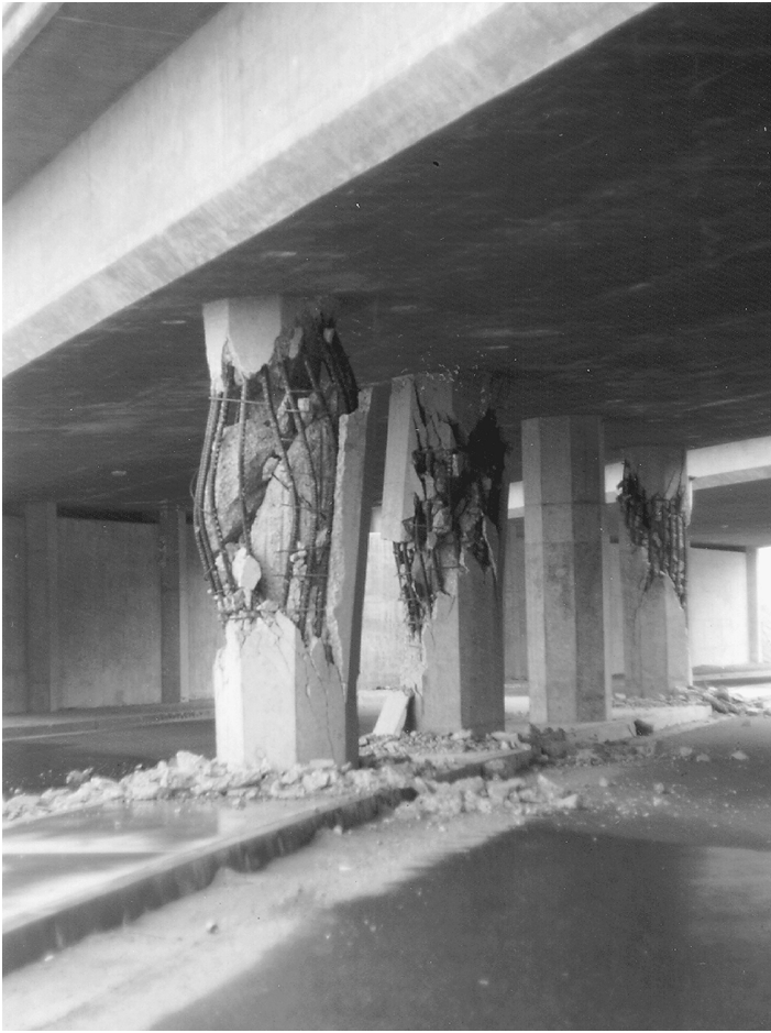
FIGURE 2.20 Failure of columns of the Route 5/210 interchange during the 1971 San Fernando earthquake.
