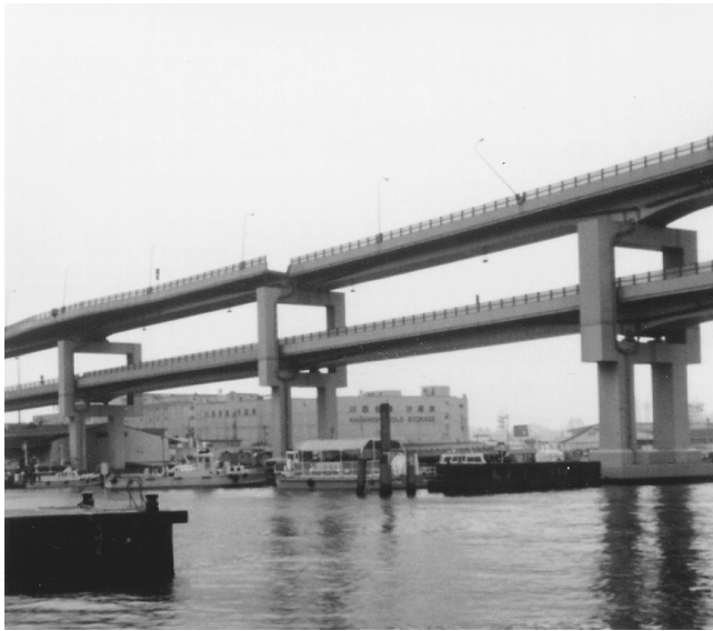
FIGURE 2.15 Hamate Bypass superstructure rotations as a result of bearing failures in the 1995 Hyogo-Ken Nanbu earthquake.
