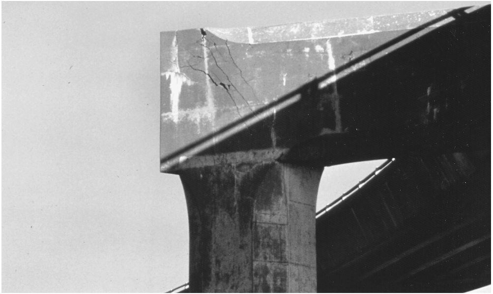
FIGURE 2.27 Outrigger damage in the 1989 Loma Prieta earthquake.
