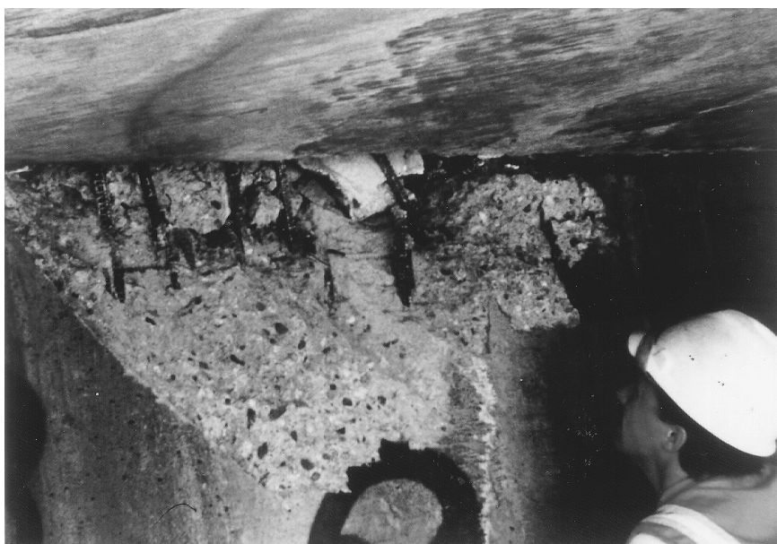
FIGURE 2.31 Damage to internal shear key in an abutment in the 1994 Northridge earthquake. (Source: EERI, Earthquake Spectra , Special Suppl. to Vol. II, 1995.)
