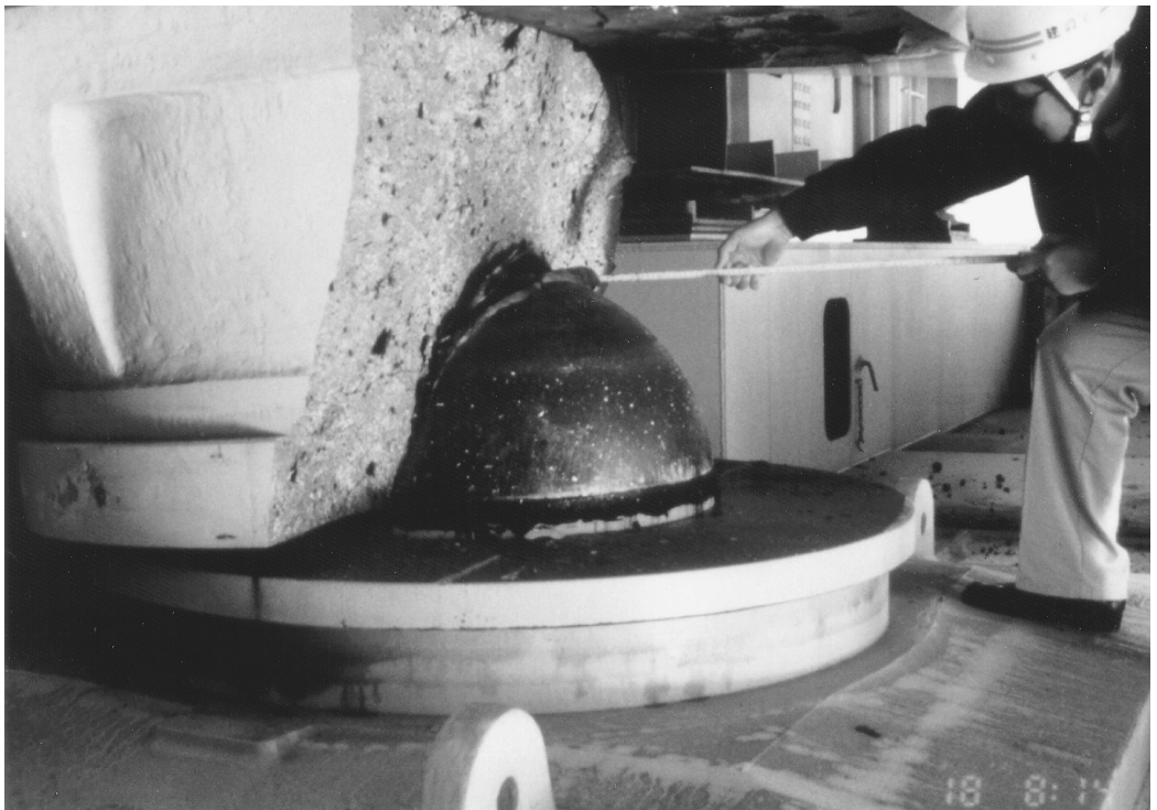
FIGURE 2.16 Nishinomiya-ko Bridge bearing failure in the 1995 Hyogo-Ken Nanbu earthquake.
