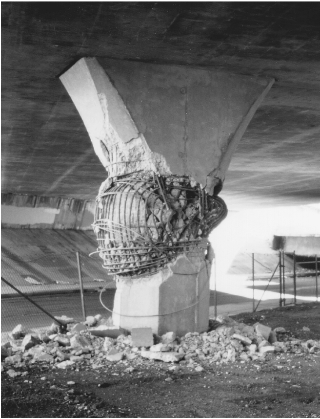
FIGURE 2.22 Failure of flared column in the Route 118, Mission-Gothic Undercrossing, in the 1994 Northridge earthquake.
