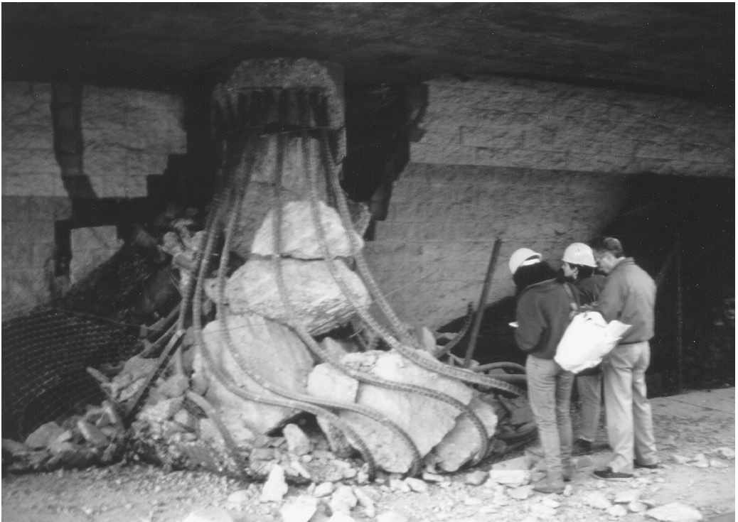
FIGURE 2.21 Failure of columns of Interstate 10, La Cienega-Venice Undercrossing in the 1994 Northridge earthquake. (Masonry walls of storage units are supporting the collapsed frame.)
