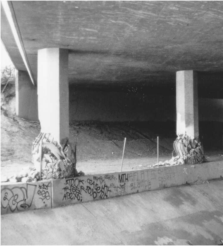
FIGURE 2.5 Bull Creek Canyon Channel Bridge damage in the 1994 Northridge earthquake.
