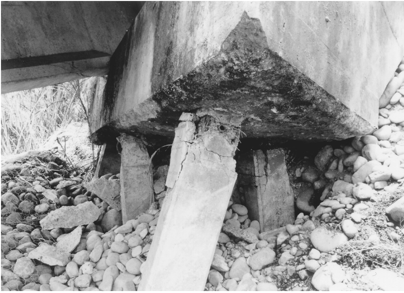
FIGURE 2.33 Abutment piles damaged during the 1991 Costa Rica earthquake. (Source: EERI, Earthquake Spectra , Special Suppl. to Vol. 7, 1991.)
