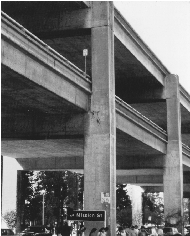
FIGURE 2.28 Embarcadero Viaduct damage during the 1989 Loma Prieta earthquake.
