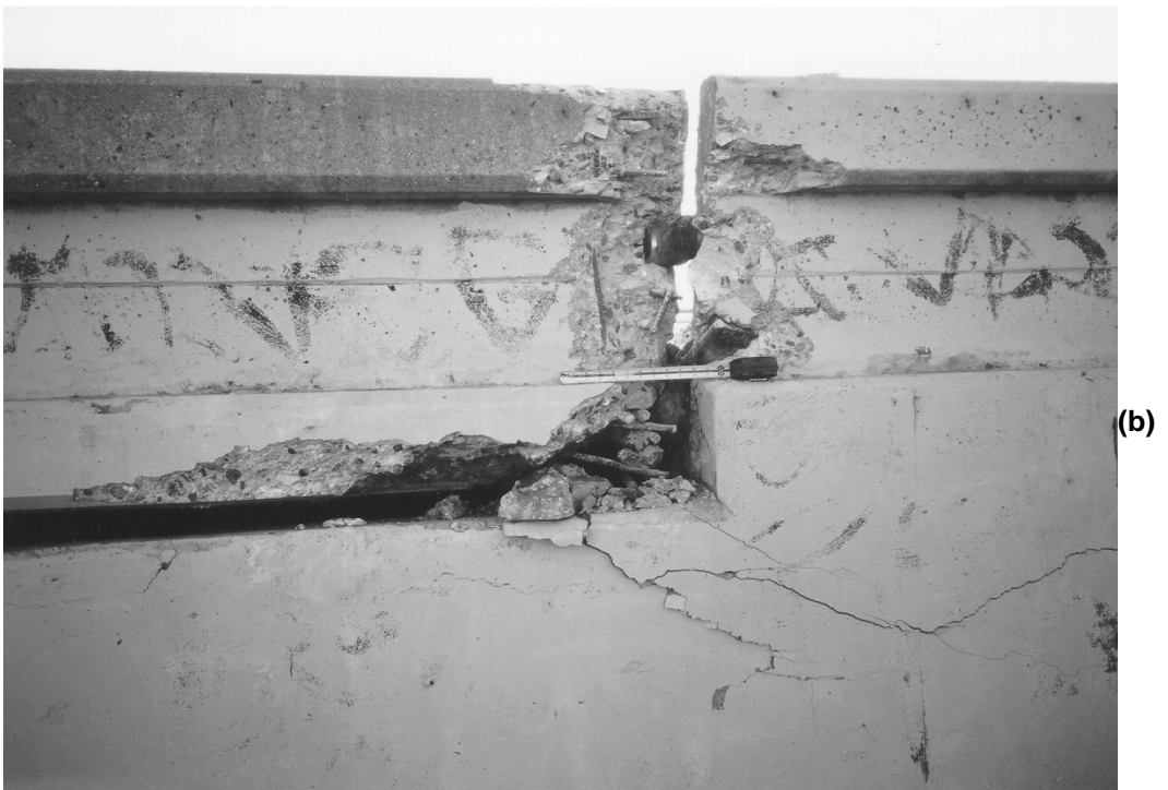
FIGURE 2.11 Santa Clara River Bridge pounding damage in 1994 Northridge earthquake. (a) Barrier rail pounding damage; (b) abutment pounding damage.
