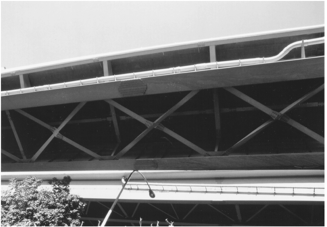
FIGURE 2.12 Buckling of braces near Pier 209 of the Hanshin Expressway in the 1995 Hyogo-Ken Nanbu earthquake.
