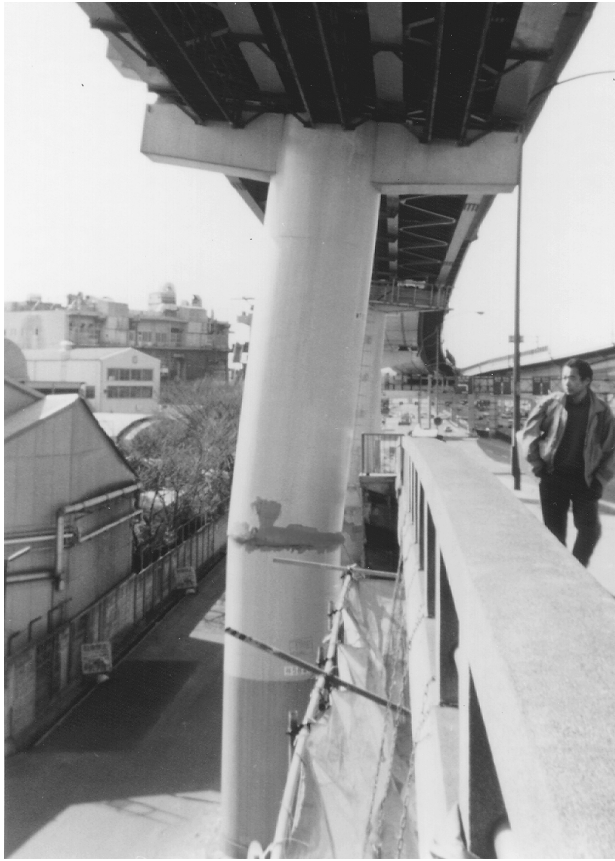
FIGURE 2.25 Local buckling of a circular cross-section column of the Hanshin Expressway in the 1995 Hyogo-Ken Nanbu earthquake.
