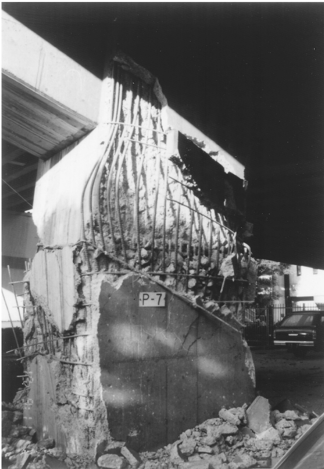
FIGURE 2.19 Failure of column with longitudinal reinforcement cutoffs near midheight in the 1995 Hyogo-Ken Nanbu earthquake.
