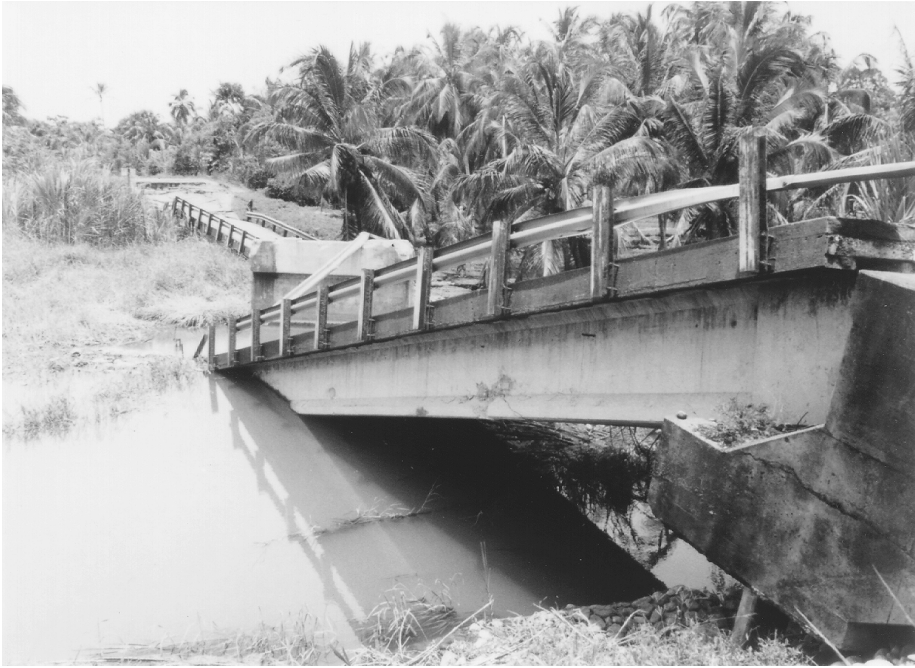
FIGURE 2.9 Rio Bananito Bridge collapse in the 1991 Costa Rica earthquake. (Source: EERI, Earthquake Spectra , Special Suppl. to Vol. 7, 1991.)
