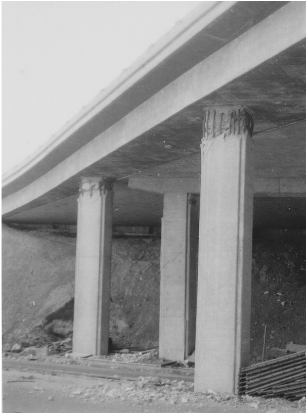
FIGURE 2.17 San Fernando Road Overhead damage in the 1971 San Fernando earthquake.
