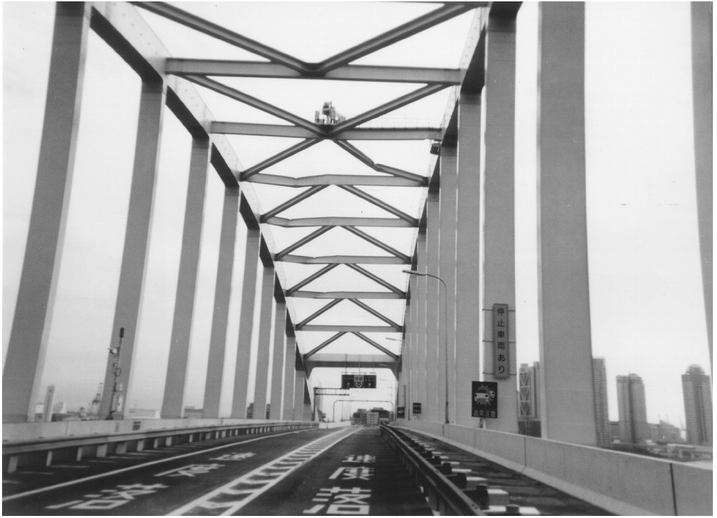
FIGURE 2.14 Buckling of cross-members in the upper chord of the Rokko Island Bridge in the 1995 Hyogo-Ken Nanbu earthquake.
