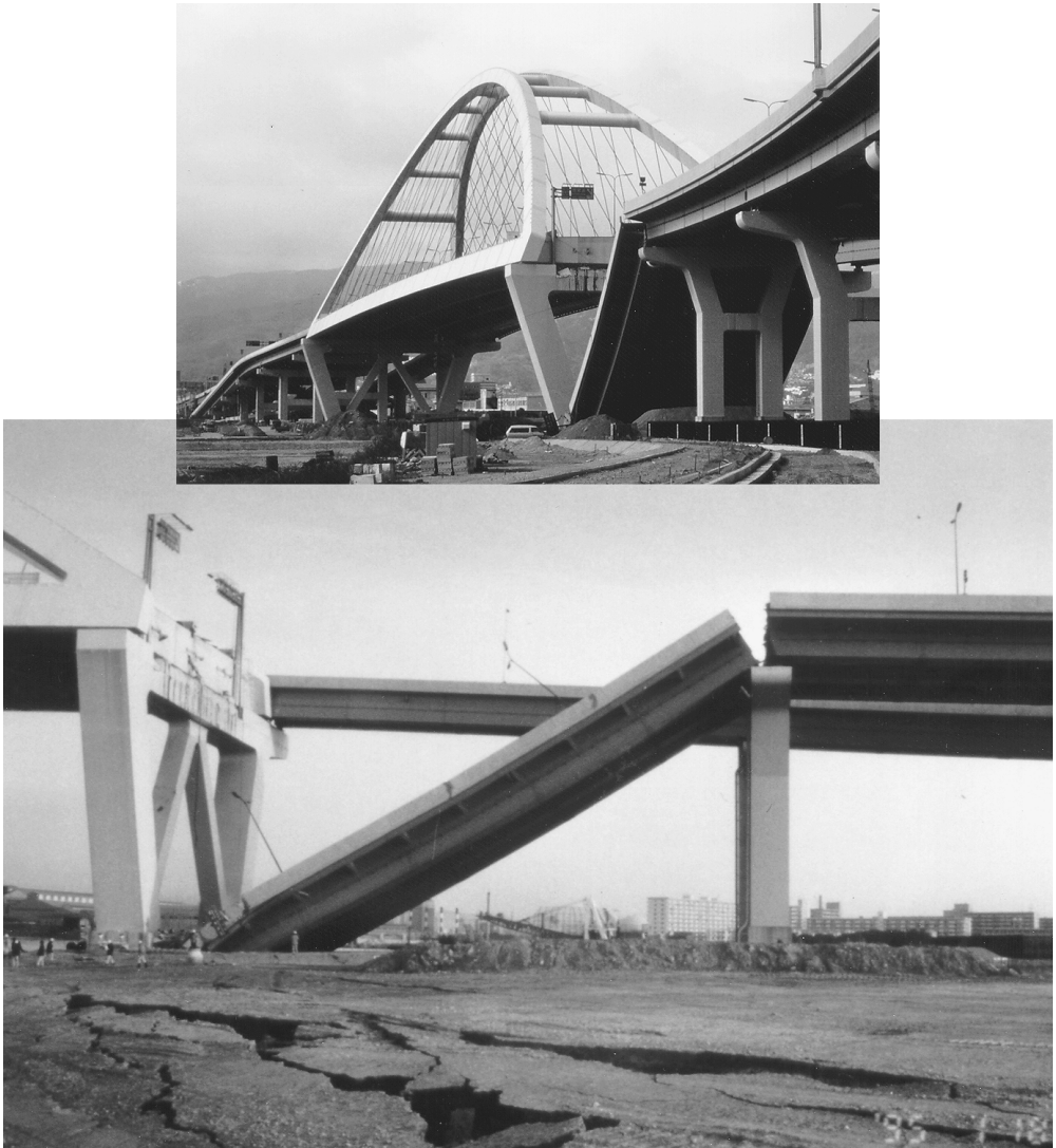
FIGURE 2.3 Nishinomiya-ko Bridge approach span collapse in the 1995 Hyogo-Ken Nanbu earthquake (Kobe Collection, EERC Library, University of California, Berkeley).
