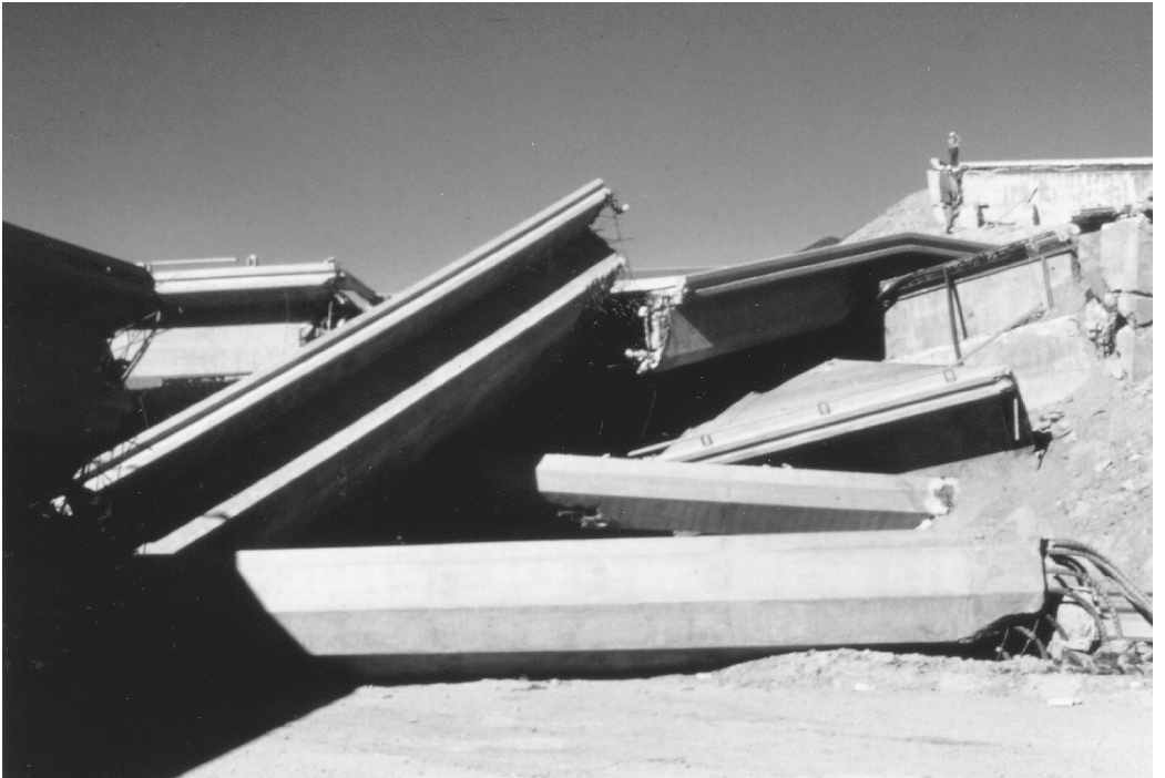
FIGURE 2.24 Failure at the base of a column supported on a single cast-in-place pile in the 1971 San Fernando earthquake (Steinbrugge Collection, EERC Library, University of California, Berkeley).
