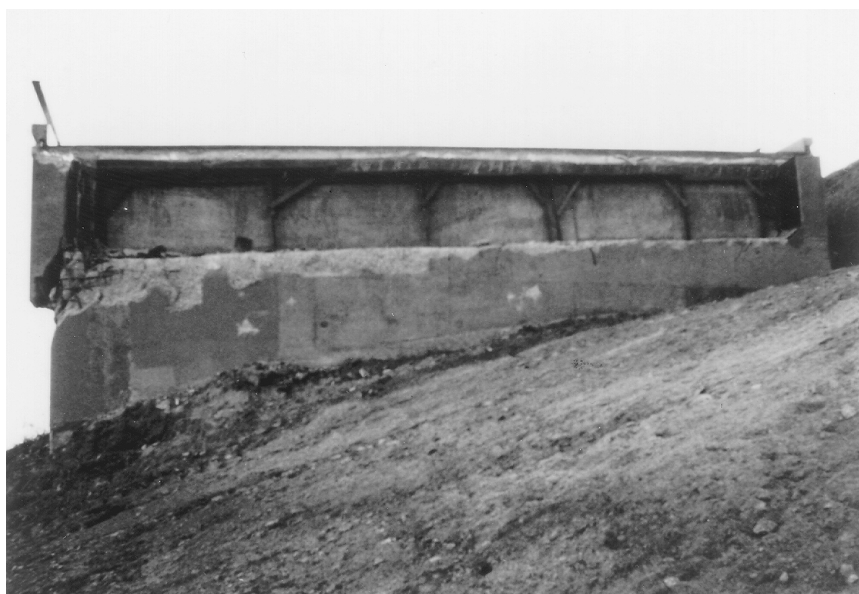
FIGURE 2.30 Damage to external shear key in an abutment in the 1994 Northridge earthquake. (Source: EERI, Earthquake Spectra , Special Suppl. to Vol. II, 1995.)
